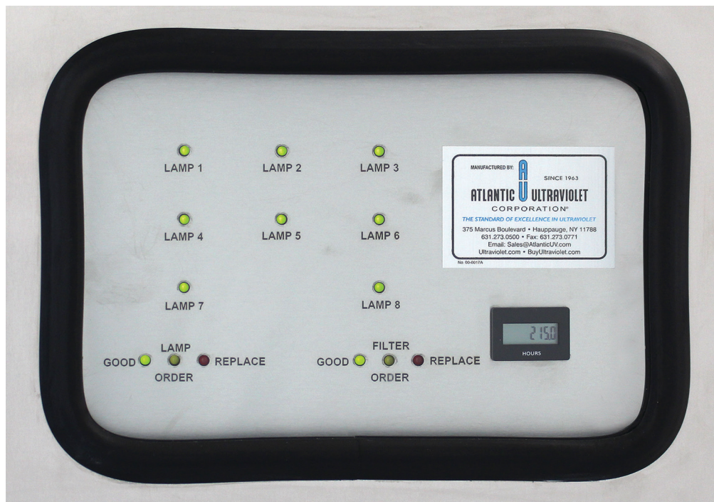
Figure 3 – SANITAIRE ® RSM2680 Monitoring Panel with All Lamps Operating Correctly
