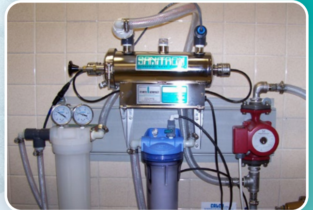
Deionizing System in Hanover Park, Illinois
