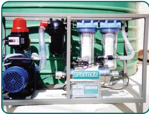
Water Purification Skid, Angola
