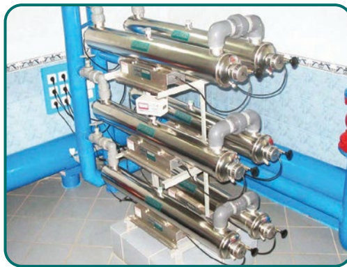
SANITRON® S15,000C Installed for Industrial Process Water
