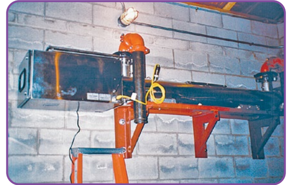
Process and Potable Water
