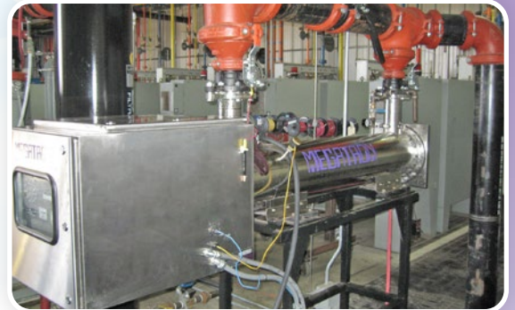
Process Water in Ohio Manufacturing Plant
