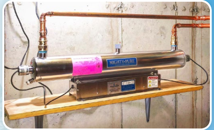
Red Hook Plumbing
