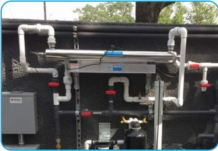
Commercial System in Windsor, California
