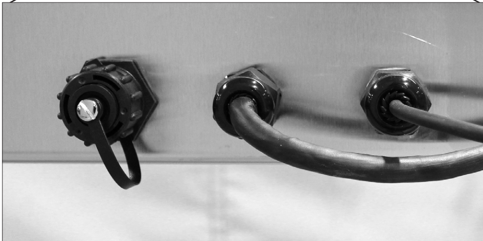
Closeup of Monitor Input and Power Line In
